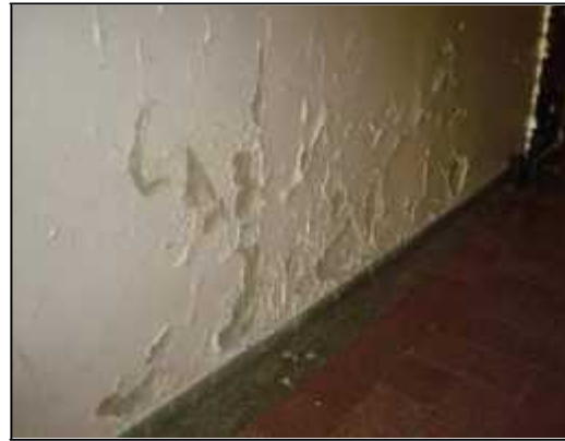
Interior view of damp penetration in the hallway
